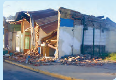
Earthquake damage in Angol.
