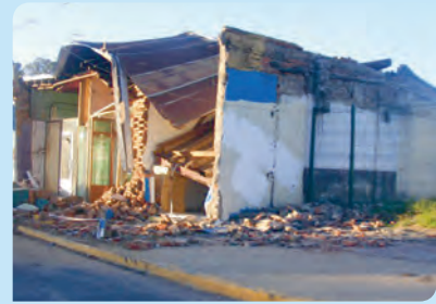
Earthquake damage in Angol.
